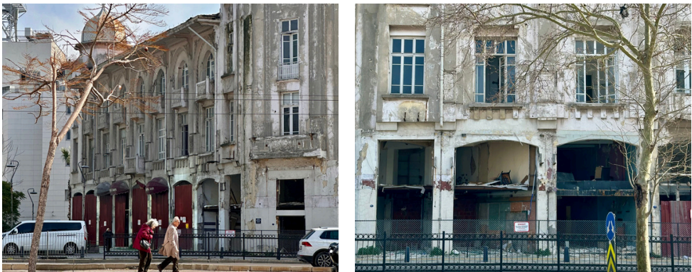
Image 3. The deteriorating facades of the Büyük Kardiçalı Han (Author, 2024).
